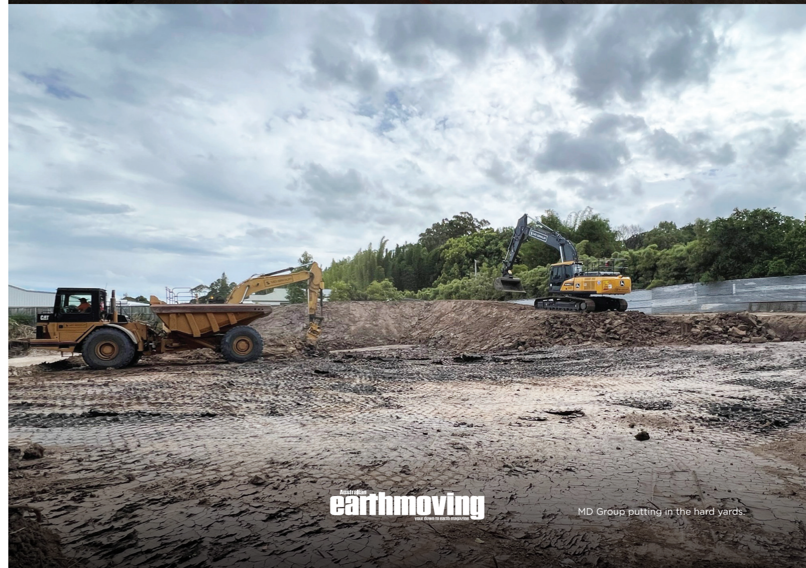
MD Group getting stuck in during their earthworks and stormwater project in Yandina.
